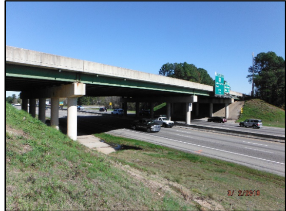
Photo 1 – View of the subject bridge, S-40-757 (Harbison Blvd) Bridge over I-26 looking up-station (Westward).
